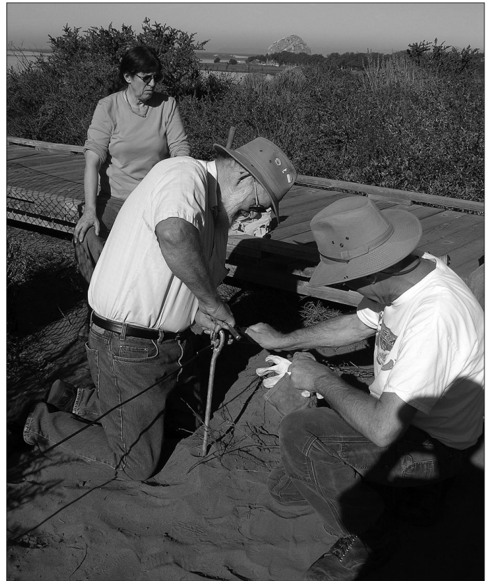
Above: Weed Warriors Bob Meyer and Henry Tate (L-R) fastened cable to a symbolic fence stanchion along the 15th Street trail while Pam Tate (far left) observed the process. Photo by Jean Wheeler.
