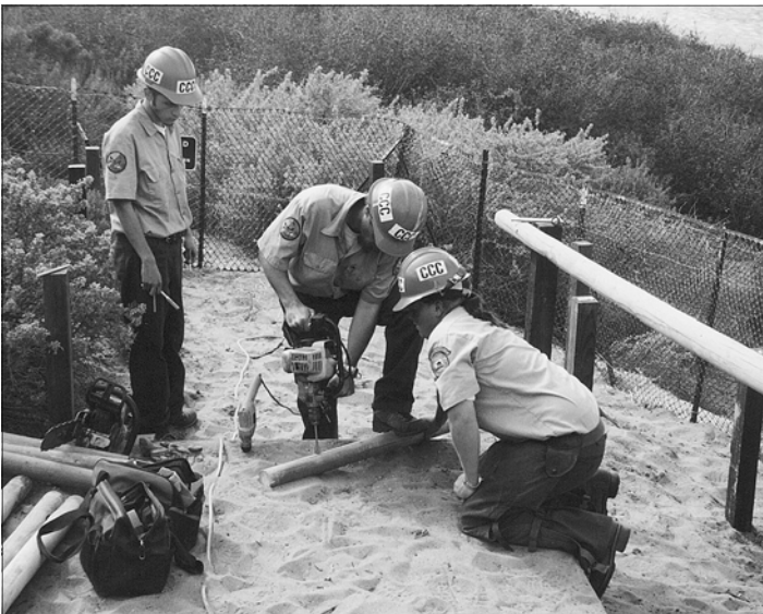
CCC Corpsmembers John Pike, Sam Hunt and Jennifer Elsea constructed wood fencing along the path Bush Lupine Point, completing the construction phase of the Elfin Forest Restoration Project. Photo by Yolanda Waddell.
