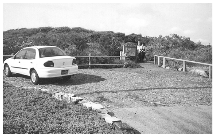
Photo above: A California Conservation Corps crew worked fast and efficiently to erect a round rail fence along the southern edge of the Elfin Forest between 11th and 12th Streets. Photo by Yolanda Waddell.
