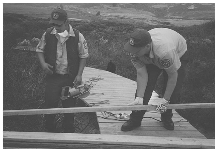
CCC Cadets Thomas Contreras (left) and Joe McNutt cut boards to length as the boardwalk loop nears completion
