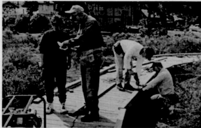
Volunteers installing "toe-rails" along the boardwalk: from l to r - Jan DiLeo, Co. Parks Planner; Paul Wolff; Keith Wimer; Pete Sarafian, SWAP Board Member
